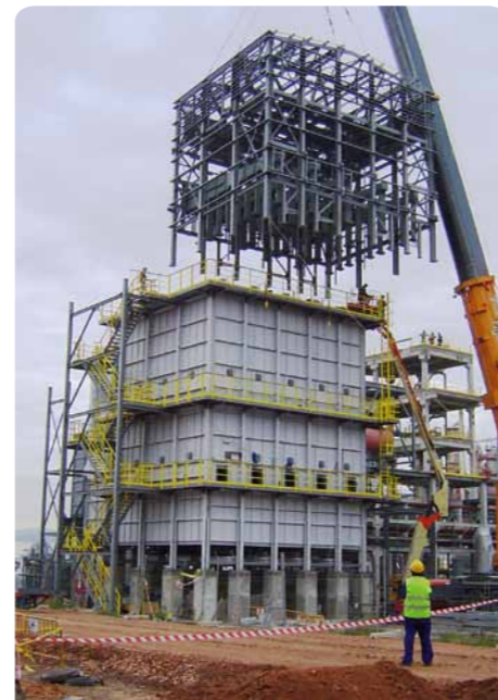
BP OIL REFINERIA Location: Castellon (ES) Tonnage: 450 Client: Technip Benelux
